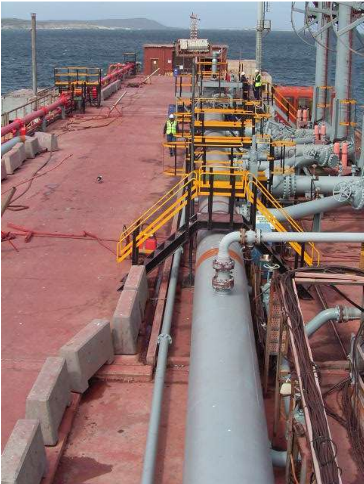
Photograph 8: View of the Jetty - Existing loading arms used for receiving of crude oil.
