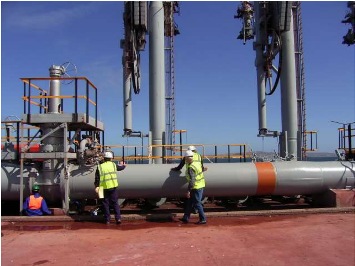
Photograph 7: View of the Jetty - Existing loading arms used for receiving of crude oil.
